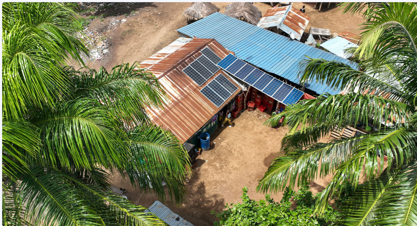
A Solergie solar panel installation in Togo. Credit: Solergie
