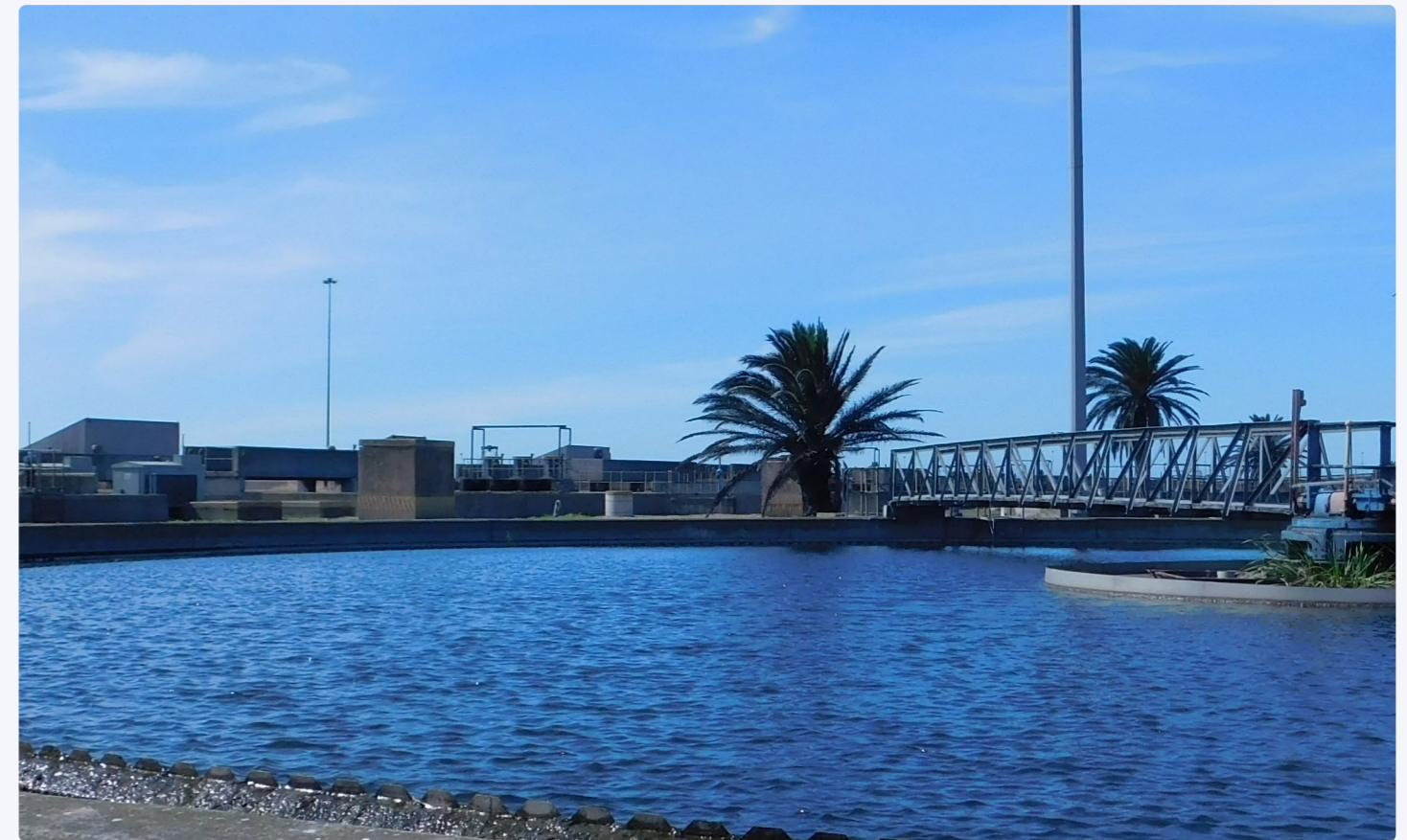
The Fishwater Flats Waste Water Treatment Works in Nelson Mandela Bay Metropolitan Municipality. The project helped the municipality install an energy metering system to better monitor the energy use and functioning of some of the plant's key assets. Credit: Charles Meadows for REEEP
