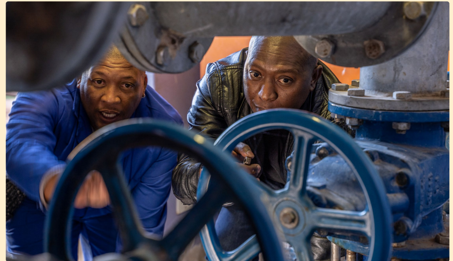
Desmond Dolopi and Derrick Bromkamp (Water Operator Kheis Municipality) inspect newly fitted pumps at Groblershoop treatment plant. Credit: Incubate
