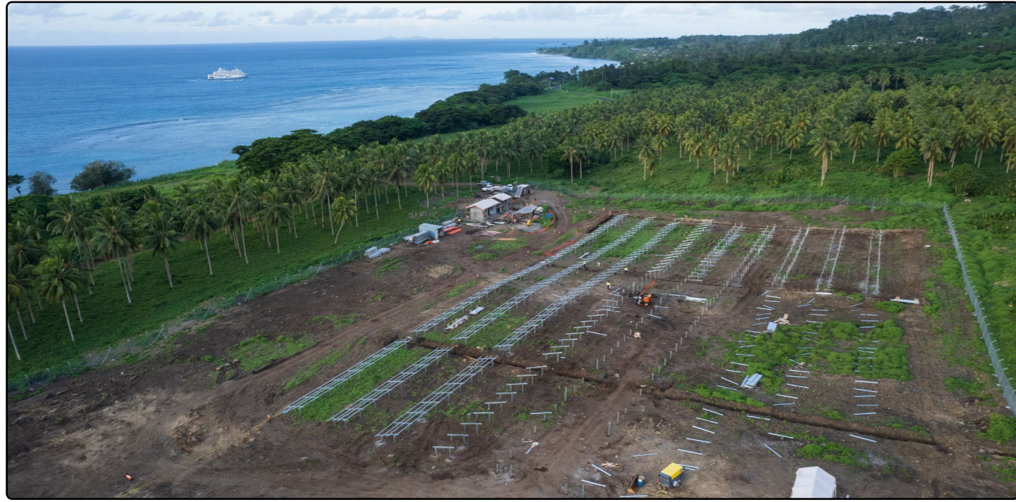
A solar panel installation in process on the island of Tavenui, Fiji. Credit: Jason Chute
